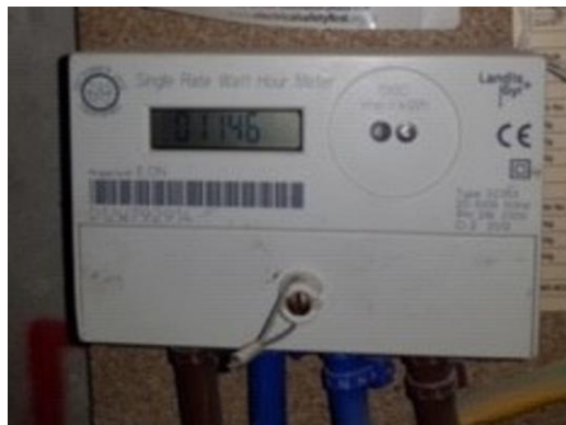
Electric meter reading
