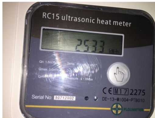
Heating meter reading
