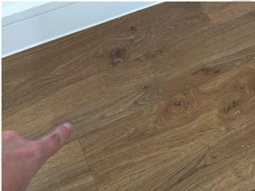
Paint splash marks on the flooring
