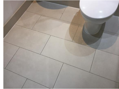
Flooring – white chemical spot stains
