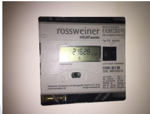
Heating Meter Reading
