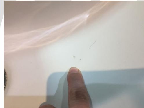
Small chip inside the sink
