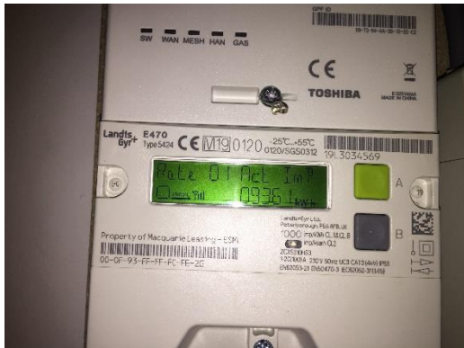
Electric Meter Reading
