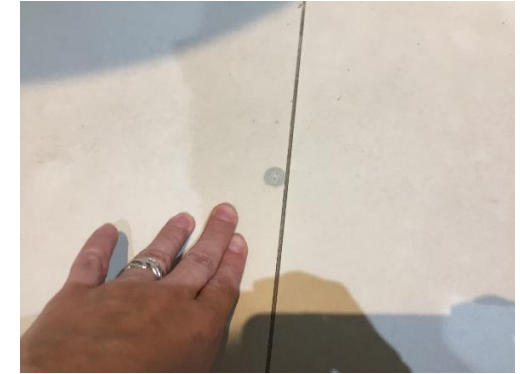
Grey paint type mark on the flooring
