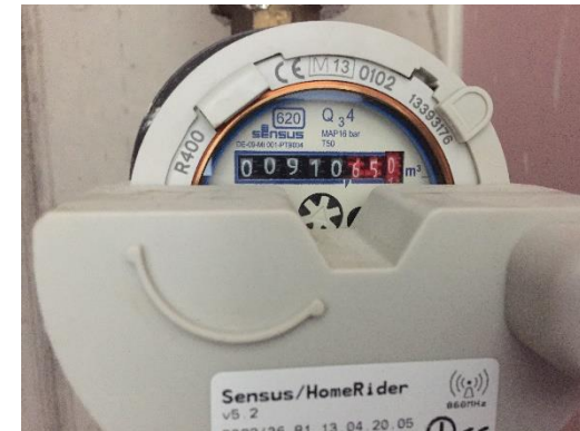
Water Meter Reading
