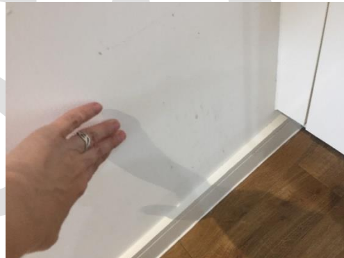
Drip marks on the wall, by the dishwasher
