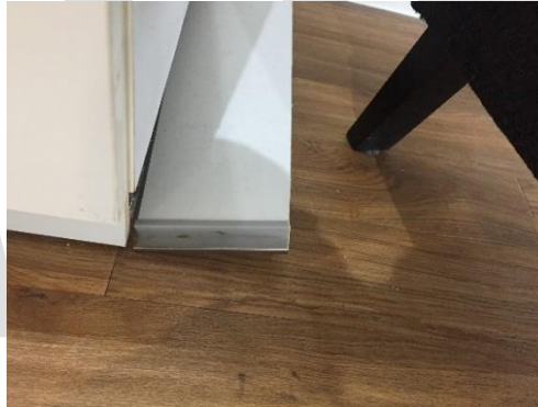
Kickboard edge panel loose
